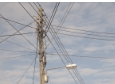
Wires in Albion Road
