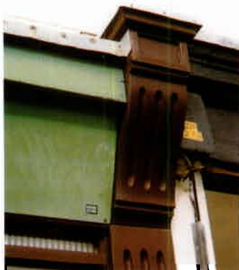
The console joins the side pilaster, both are routed vertically
