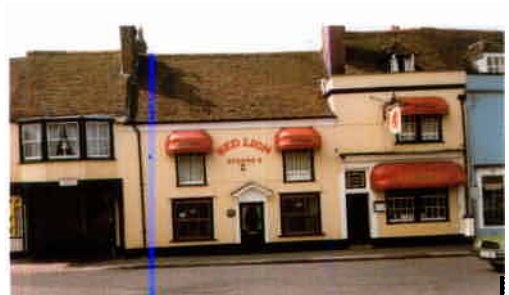
Inappropriate use of non traditional, fixed plastic blinds. Those at high level look particularly awkward.
