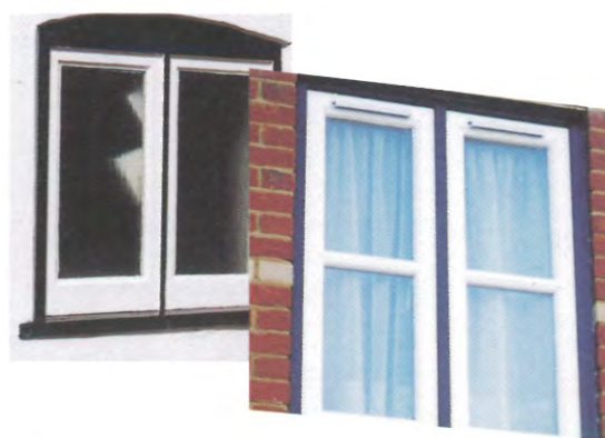
A traditional decorative effect on old and new joinery - the window frame contrasts with the tone of the opening casement.▲
