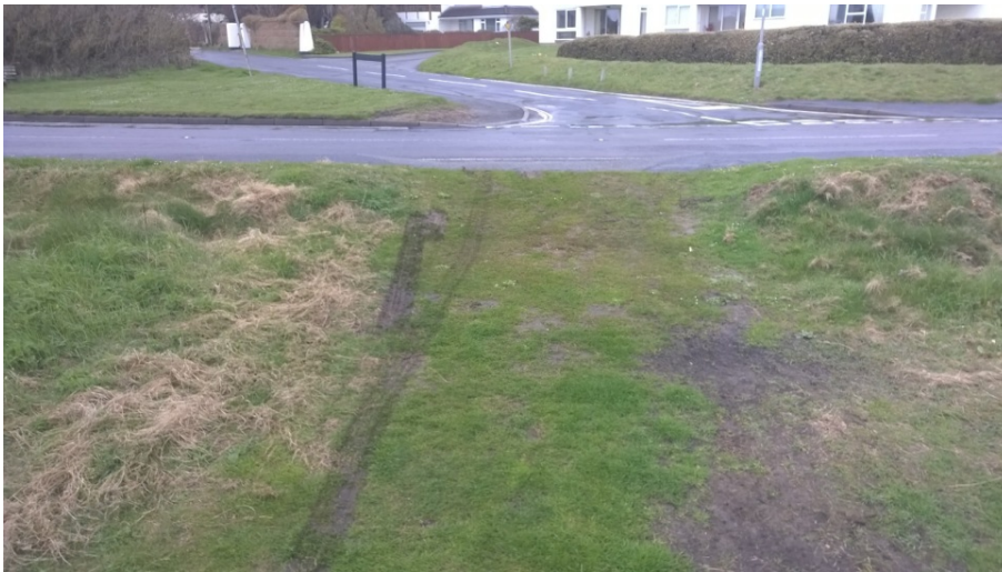
Figure 2 - Area showing pedestrian and unauthorized vehicle incursion damage
