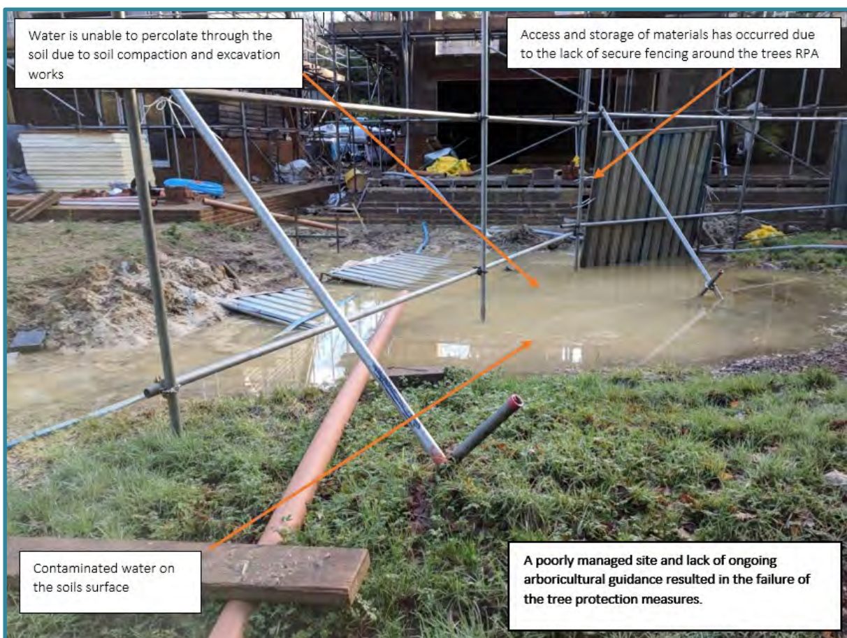
Figure 21. Failure to protect trees to be retained
