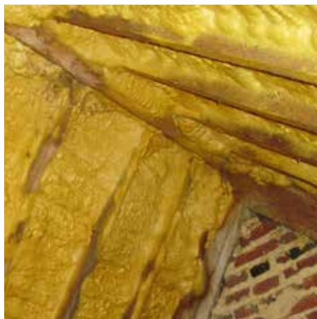
Inappropriate use of foam sealant
