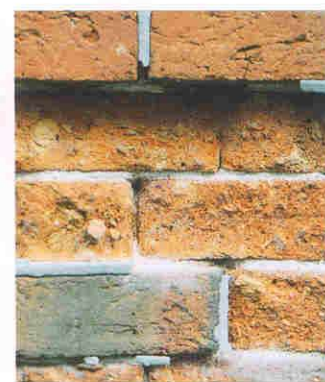
Damaging effects of cement mortar
