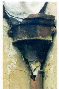
Poor detailing & broken cast iron downpipe
