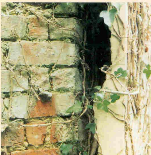
Failed cement render
