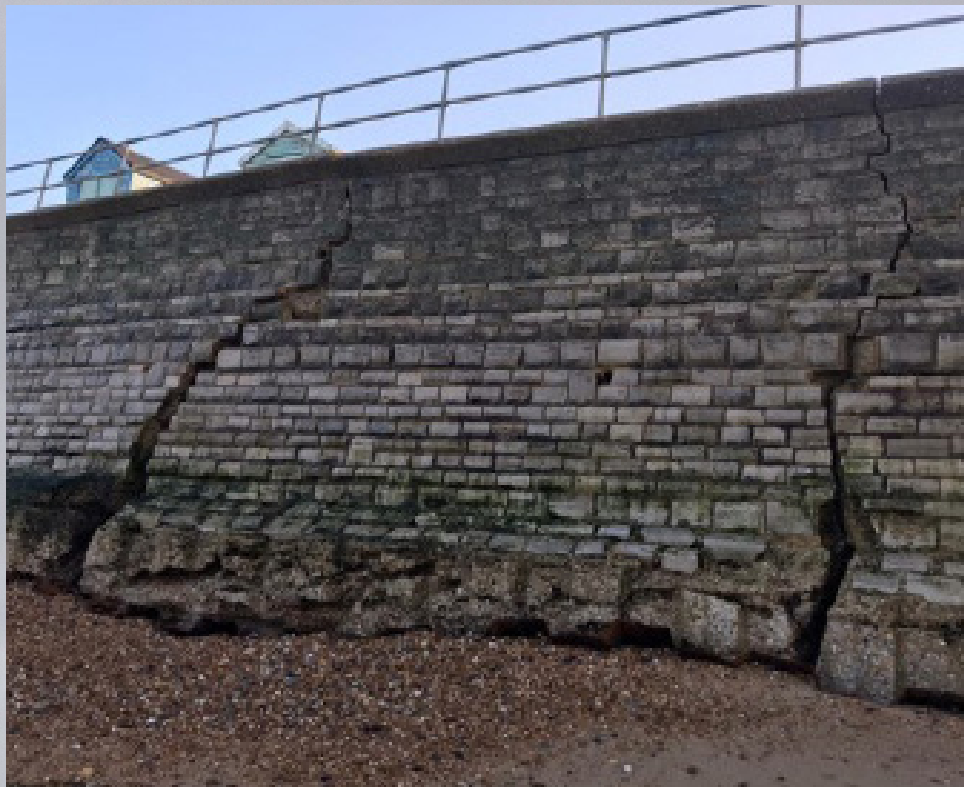
Major cracks in the seawall
