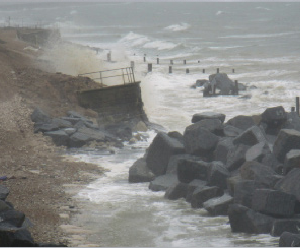
Failed Seawall at Milford
