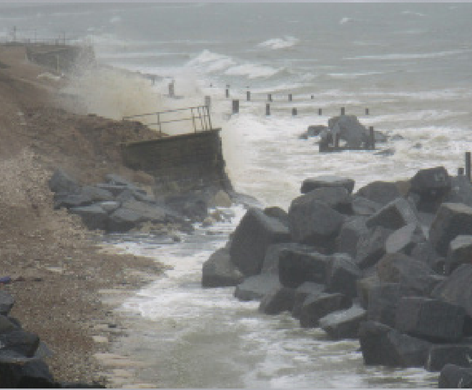
Failed Seawall at Milford
