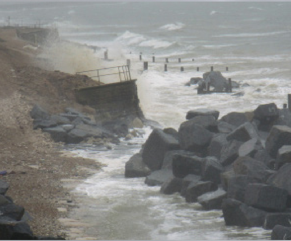
Failed Seawall at Milford
