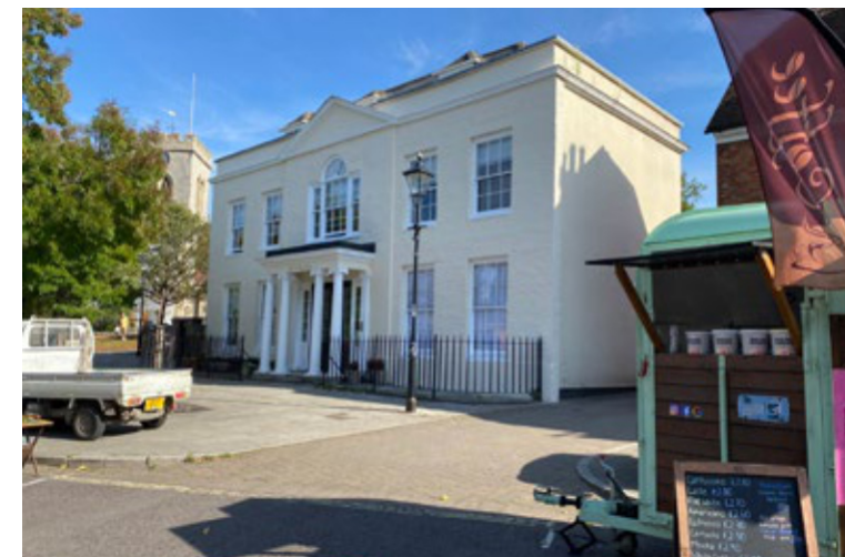
6. Upgrade in paving required
