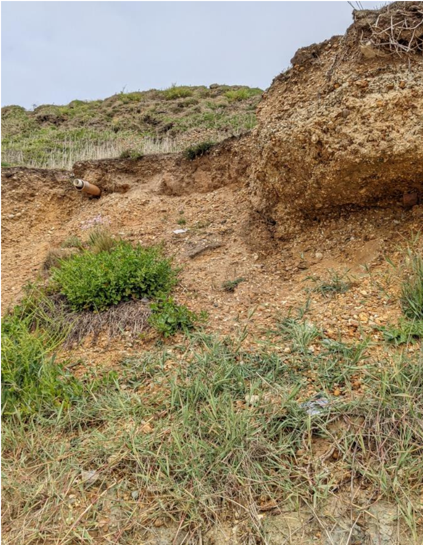
Figure 0-18 Photo of earlier failure showing pipe, cemented overhang and water line. Photo taken 07/06/2022. Approx. Ordnance Survey grid reference SZ 27757 91743.
