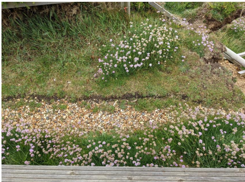
Figure 0-11 Photo of crack, taken 07/06/2022. Approx. Ordnance Survey grid reference SZ 27755 91751.
