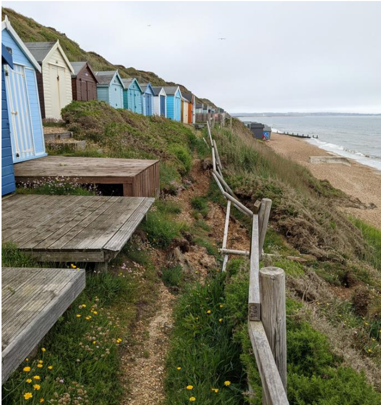
Figure 0-12 Photo of western cliff slump. Photo taken 07/06/2022. Approx. Ordnance Survey grid reference SZ 27709 91766.
