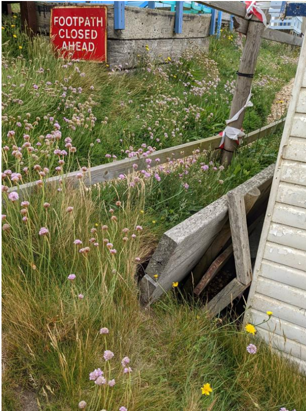
Figure 0-5 Example of failed slope retention at the beach huts along the beach. Photo taken on 07/06/2022. Approx. Ordnance Survey grid reference SZ 27649 91790.
