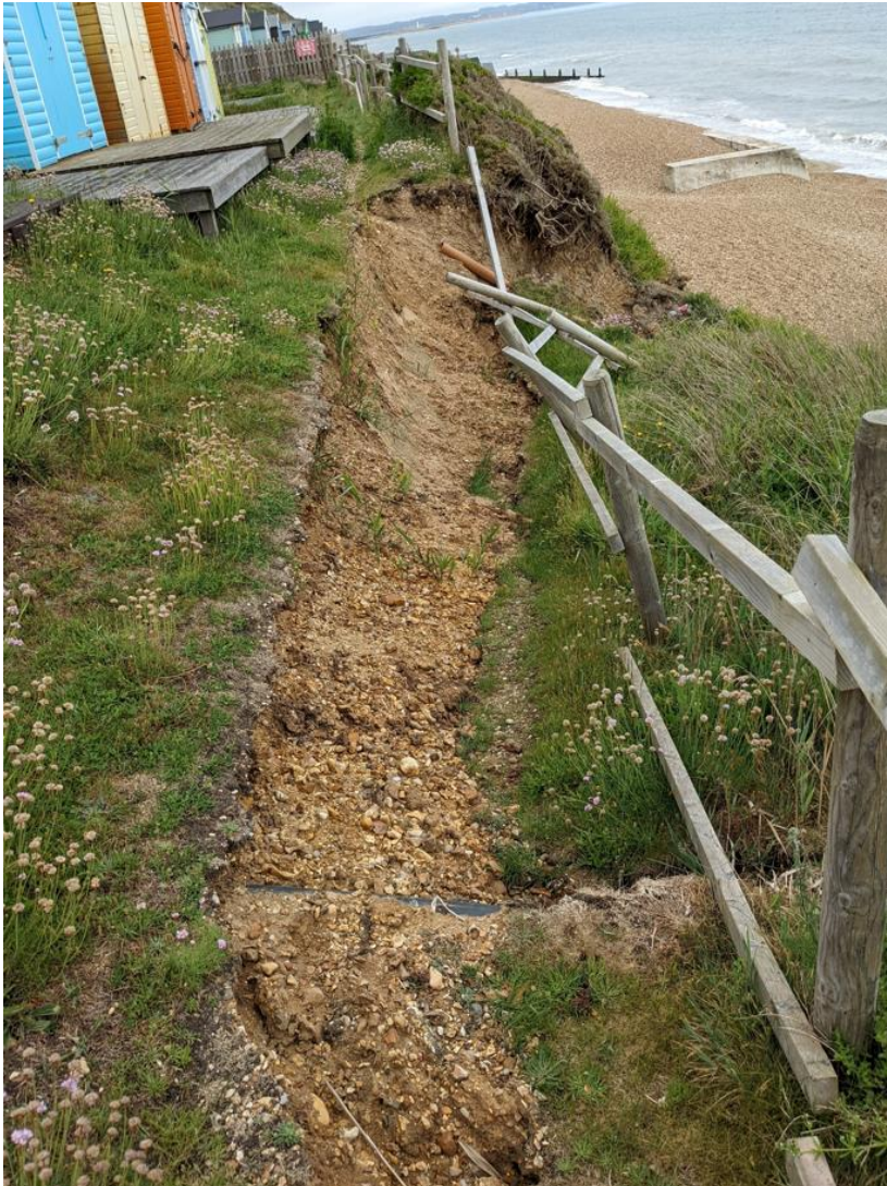
Figure 0-16 Photo of second cliff slump. Photo taken 07/06/2022. Approx. Ordnance Survey grid reference SZ 27732 91757.
