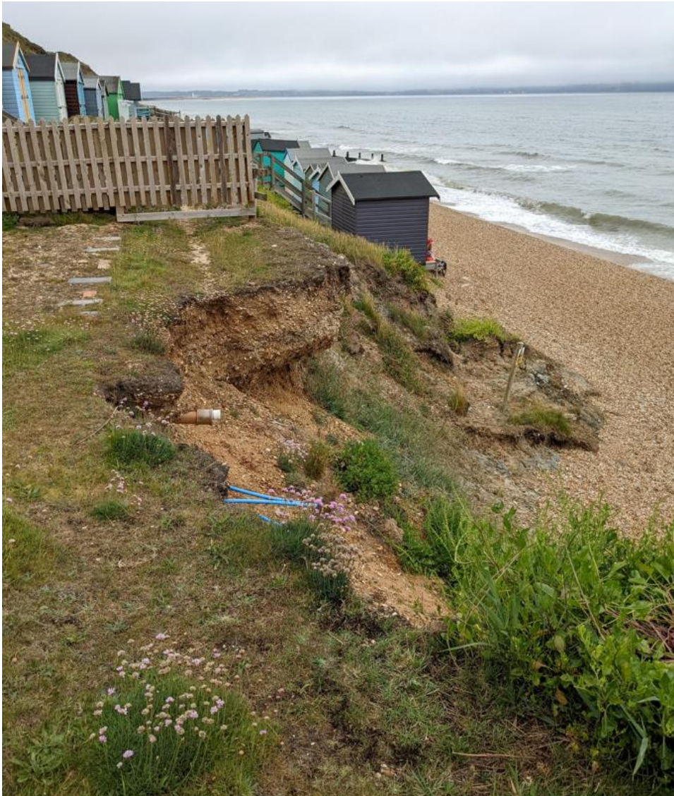
Figure 0-17 Photo of earlier failure. Photo taken 07/06/2022. Approx. Ordnance Survey grid reference SZ 27753 91752.
