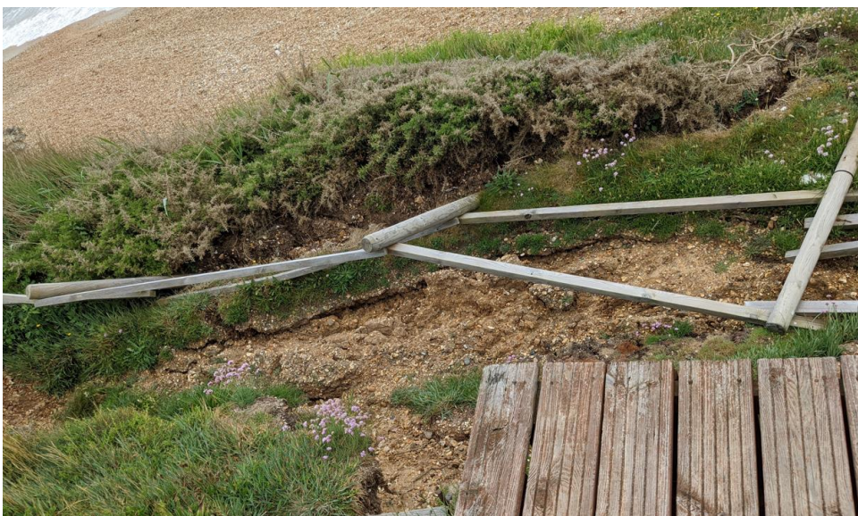
Figure 0-13 Photo of crack at the top of the western cliff slump. Photo taken 07/06/2022. Approx. Ordnance Survey grid reference SZ 27711 91767.
