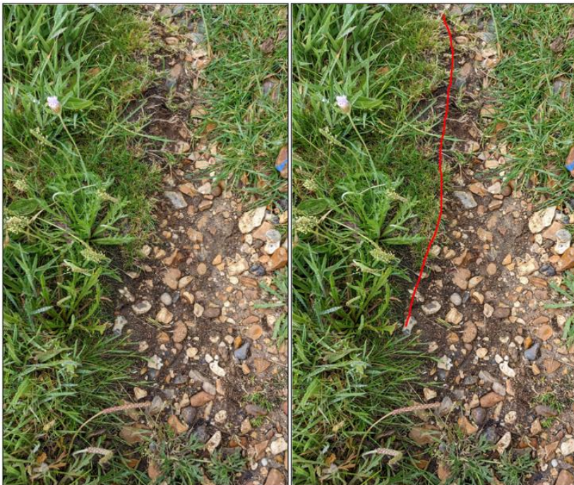
Figure 0-9 Photo of crack, taken 07/06/2022. Approx. Ordnance Survey grid reference SZ 27704 91768.
