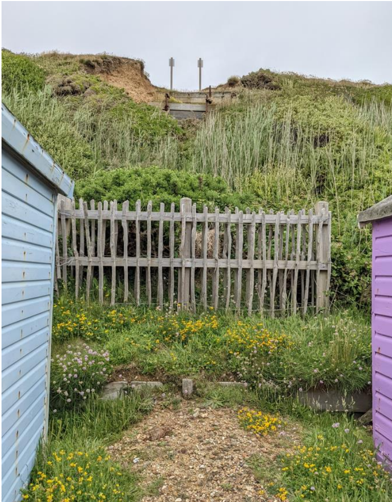
Figure 0-19 Photo of other failure higher up the slope. Photo taken 07/06/2022. Approx. Ordnance Survey grid reference SZ 27642 91794.
