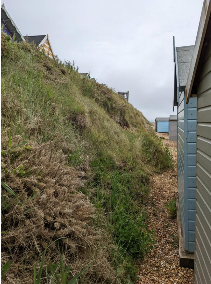
Figure 0-7 Photograph showing the slope gradient behind the beach huts on the beach. Date taken 07/06/2022. The photograph was taken behind the beach huts to the east of the area specified in the brief. Approx. Ordnance Survey grid reference SZ 27784 91733.
