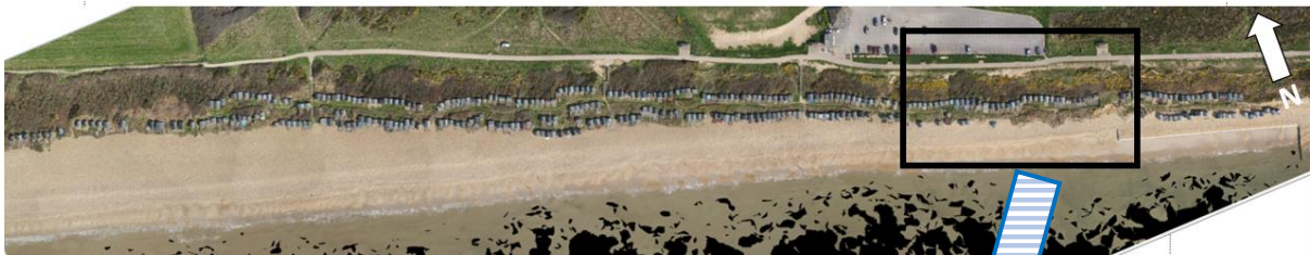
Location of beach hut damage, to eastern end of site
