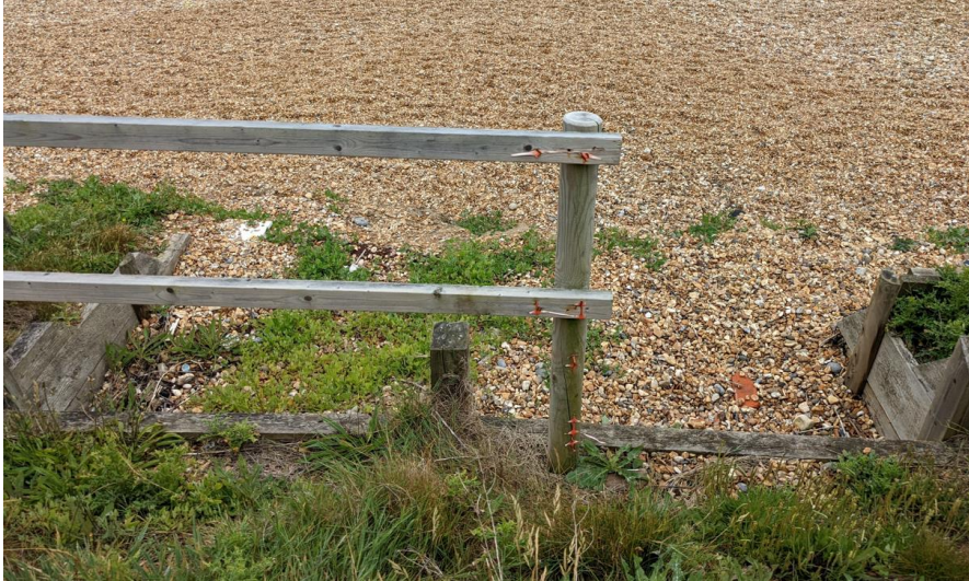
Figure 0-4 Example of how beach hut bays have removed toe of the slope and added in ad-hoc retaining structures. This beach hut has been removed due to damage from the February 2022 storms. Photo taken on 07/06/2022. Approx. Ordnance Survey grid reference SZ 27687 91768.
