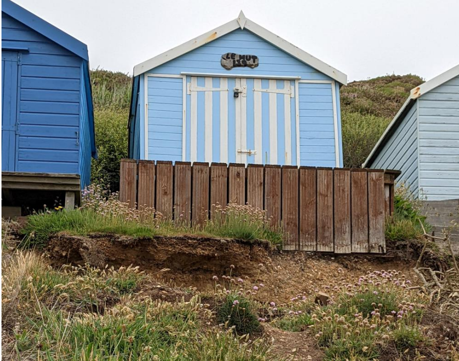
Figure 0-14 Photo of the overhang and undermining of the beach hut decking at the western cliff slump. Photo taken 07/06/2022. Approx. Ordnance Survey grid reference SZ 27708 91760.
