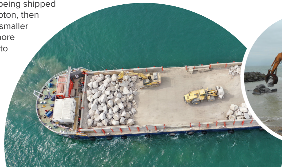
Inset image above: Damaged seawall. Images right (left to right): Rocks on the barge; Rocks being delivered from the barge; Rocks on the beach; Example of a completed revetment.
